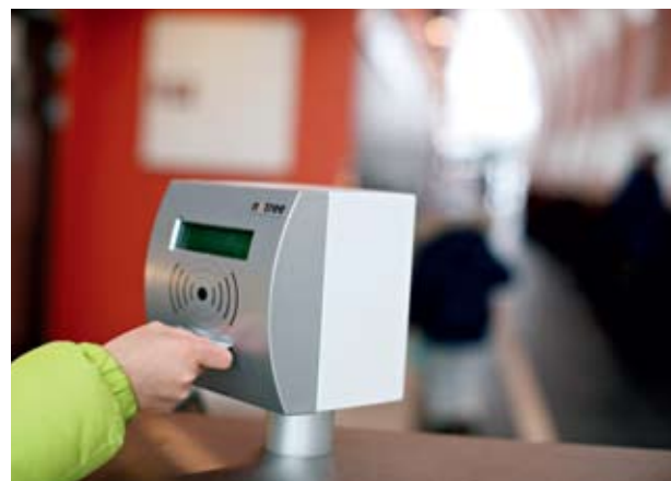
Drammensbadet has an electronic ticketing system and a system for access control that registers bar code tickets and smartcards. The electrical installations were carried out by Moelven Elektro.
